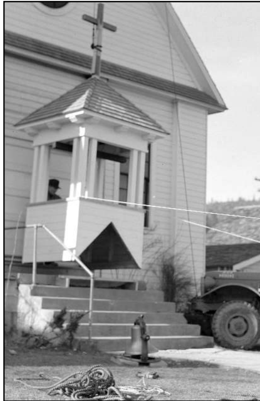
As the bell tower is lifted into place on to the roof of St. John's Church, Quincy in 1952, the bell rests on the grass below the church steps, center.
