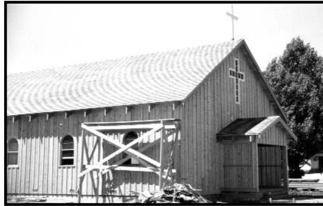
Construction nears completion of the Christ the King Church in Chester in 1955.
